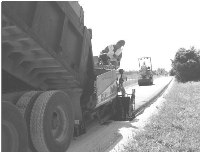
APAC was the winning bidder to complete the most recent section of paving work on the FHT into Springfield.
